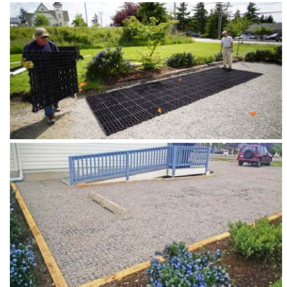
Top: Stabiligrd is placed atop a surveyed, sub-grade surface. Bottom: Gravel is placed and raked over Stabiligrd to allow water infiltration.
