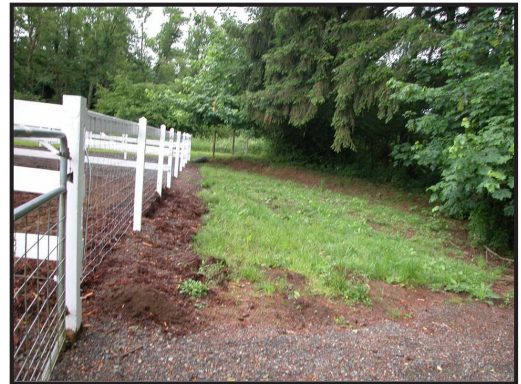
Turnouts with a grassy buffer strip allow runoff to be filtered before it enters a nearby stream.
